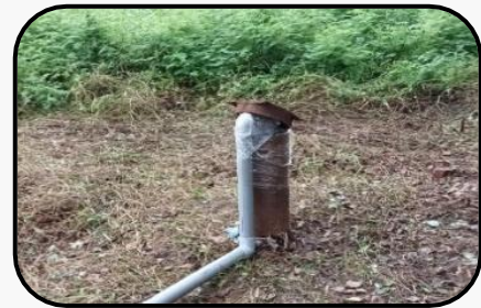
Use of unused borewells for groundwater recharge
