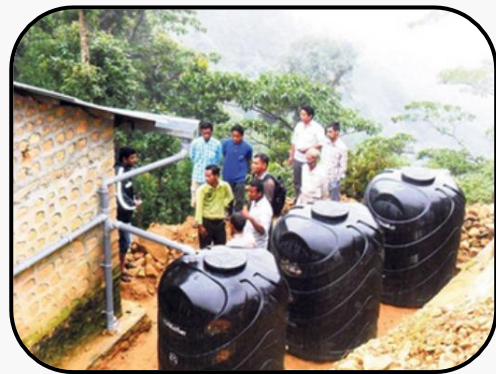
Roof Top Rainwater Harvesting
