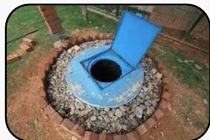
Use of drums in recharge pits
