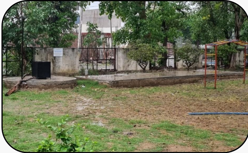
An Artificial Recharge System (Desilting Chamber, Filters and Recharge Borewell) in Faridabad
