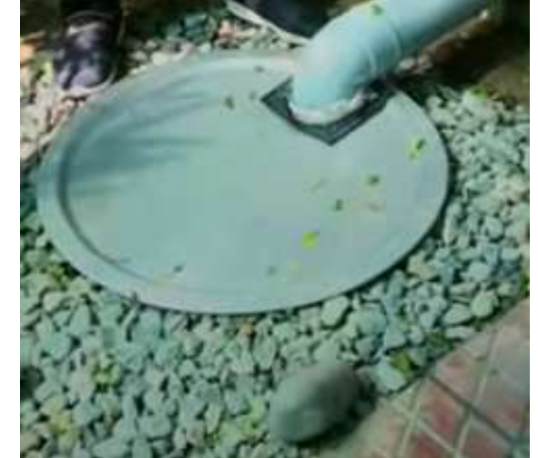
09) Fixing with Jali at top to avoid penetration of dust particles in side from top covering
