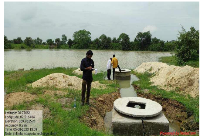
Percolation Ponds with Recharge Wells
